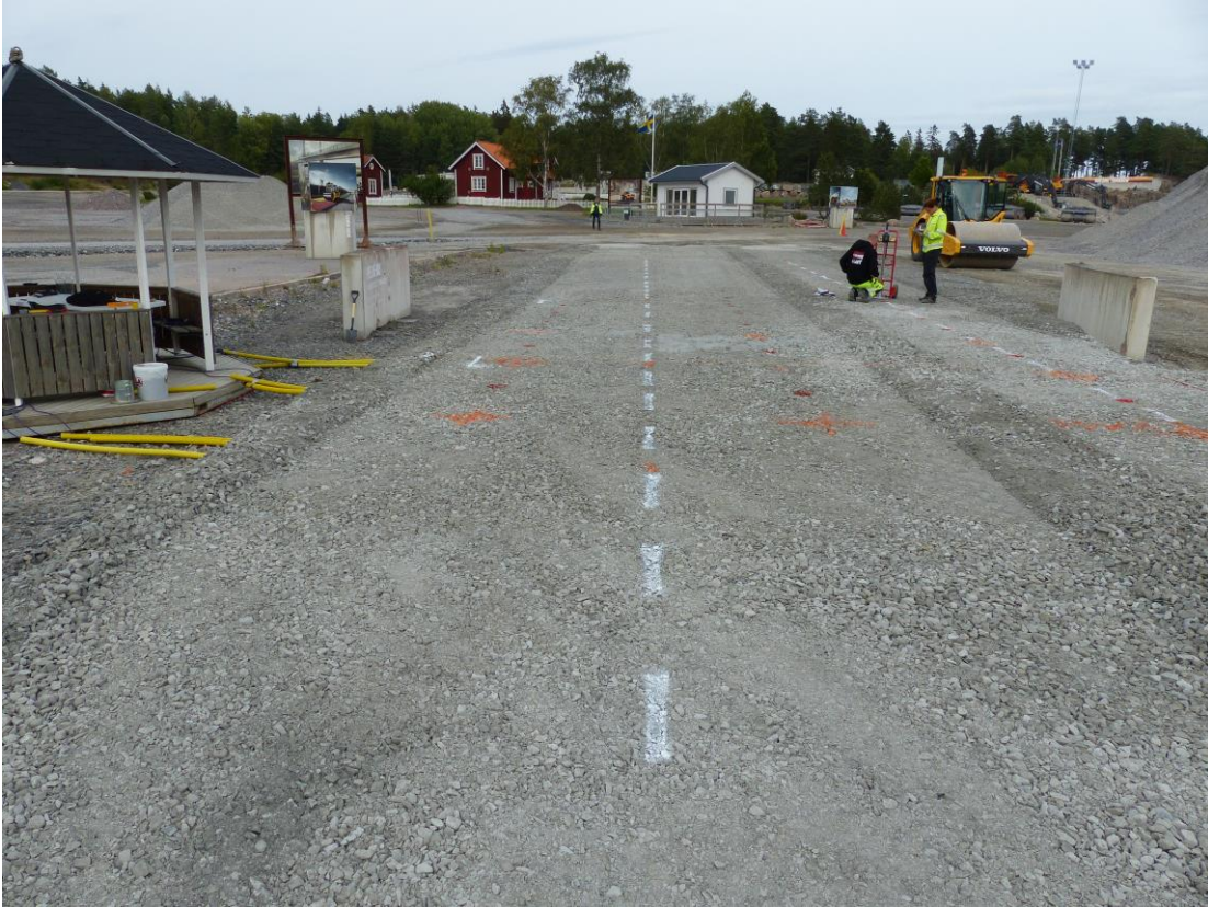
Figure 5. Photo of the test track after the first two static roller compaction passages.
