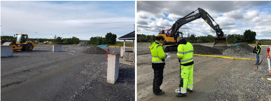
Figure 1. Left: Site after ground compaction and placement of concrete blocks used for laser scanning reference sphere positioning. right: Light deflectometer measurements and material spreading.
