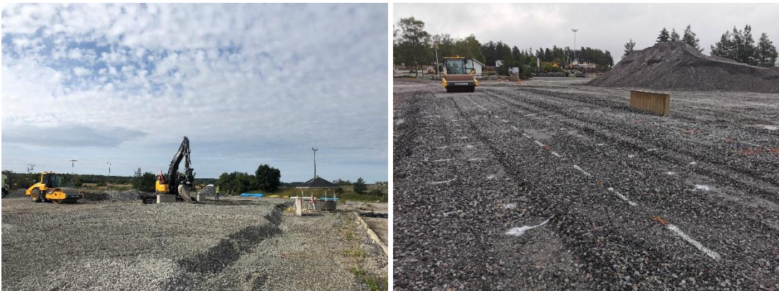
Figure 3. Left: Final adjustment of bed height using excavator and laser height measurement. Right: Tracks after completion of 64 passes before final compaction.
